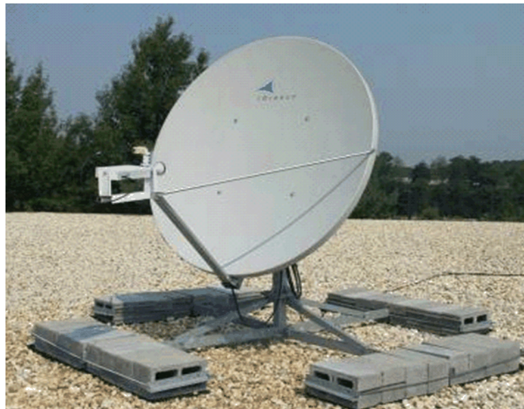
Figure 5. Typical Antenna with BUC and LNB
